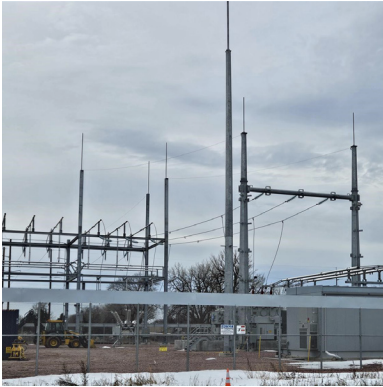
The Great Plains Substation is located in Sioux Falls, South Dakota.
